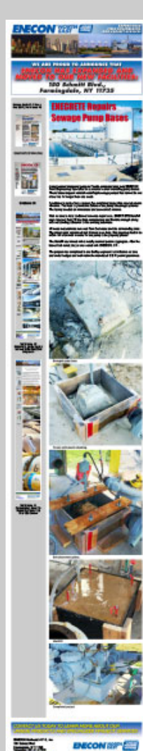
Vol 9 Issue 13 Pump Bases Rebuild With ENECON Polymers
