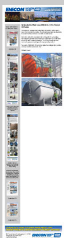
Volume 7 Issue 9 Exterior of Fuel Tank Protected with Eneseal CR
