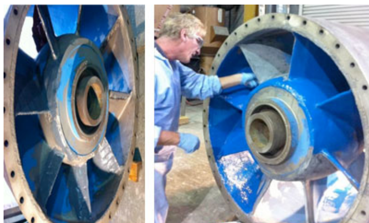
Rebuilding grade CeramAlloy CP+AC used to repair vanes. CeramAlloy CL+AC used to coat all surfaces.
