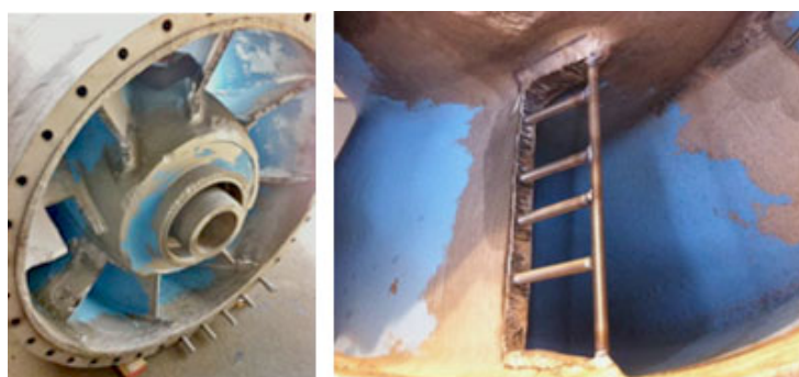
The severely eroded vanes were cut away and a threaded rod "skeleton" installed.
