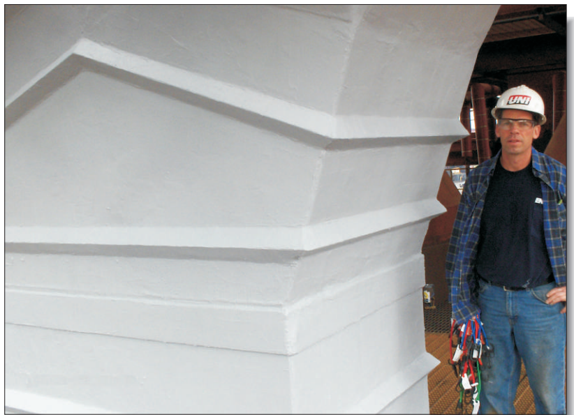
After totally encapsulating the unit in DurAlloy, ENESEAL CR was used to provide optimum corrosion resistance and a uniform look.
