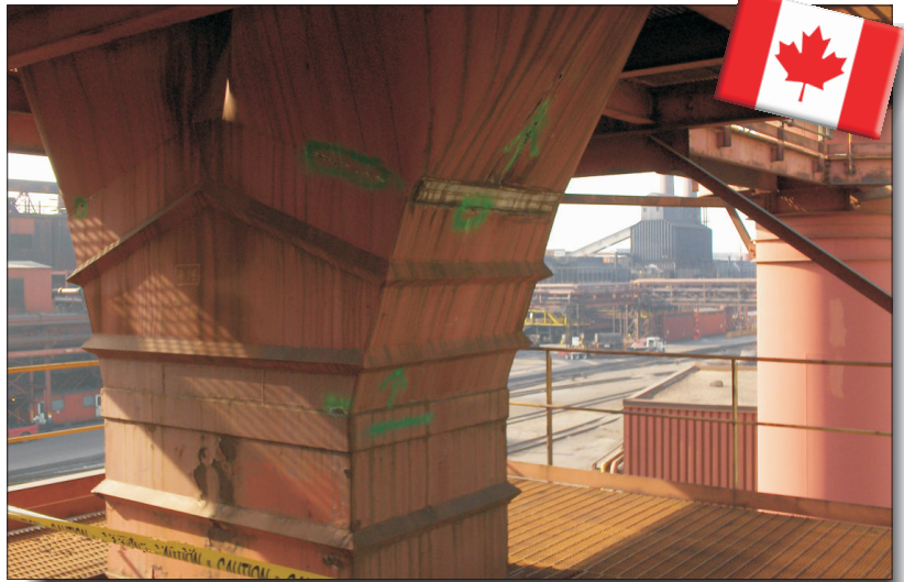
The fume extraction system.
